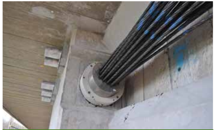
Steel Tensioning Cables
